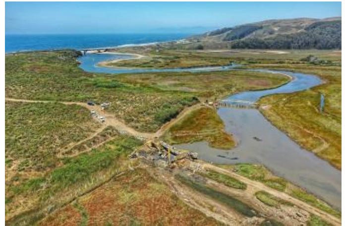
Restoration work in Pescadero Marsh. Photo courtesy of San Mateo Resource Conservation District.
